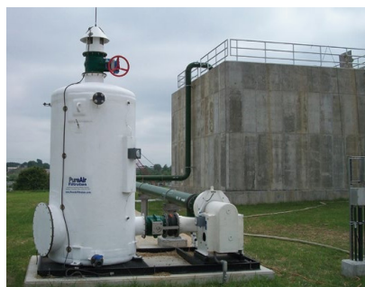
VERTICAL BED SCRUBBER
