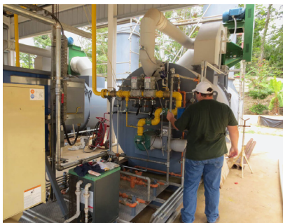
125 GAL/HR LIQUID WASTE THERMAL PLANT
